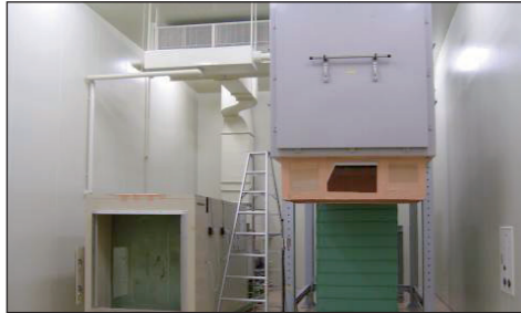
Air Volume Measurement Room
