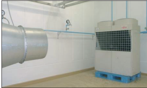
Shower Test Room
